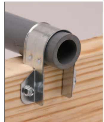
Perpendicular pipe run top mounted on wood joist
