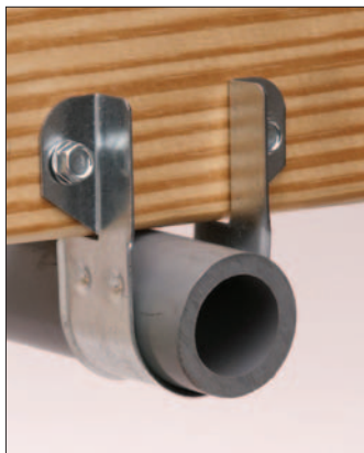
Perpendicular pipe run bottom mounted on wood joist
